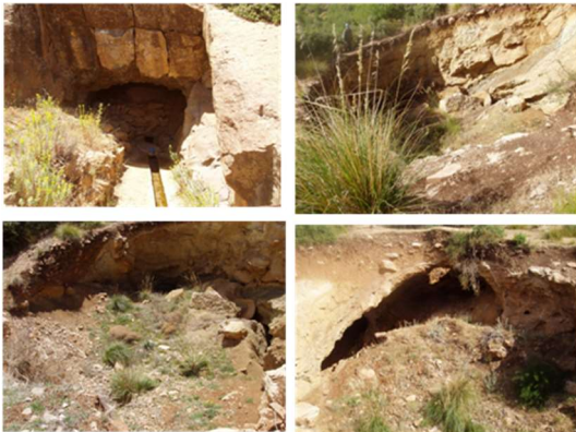
Fig. 2: Collapse cases of galleries in the Ichmoul mine site.
