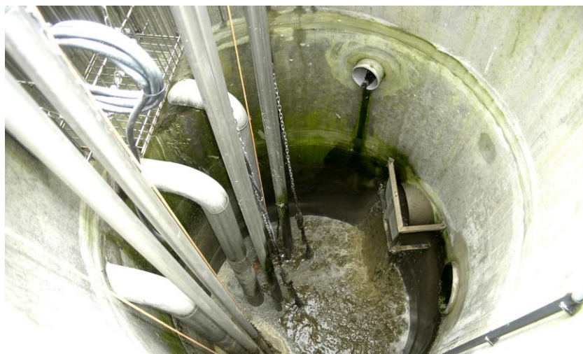
Figure 3.3: Post de pompage
