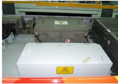
Figure 1-21: Picture of the battery box.
