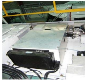
Figure 1-19: picture of the room air conditioning unit.
