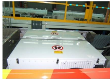
Figure 1-22: picture of the CVS static converter.
