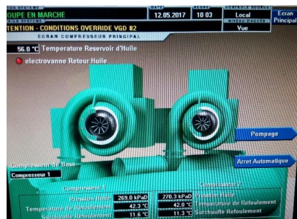
Figure 2-10 - Ecran compresseur principal
