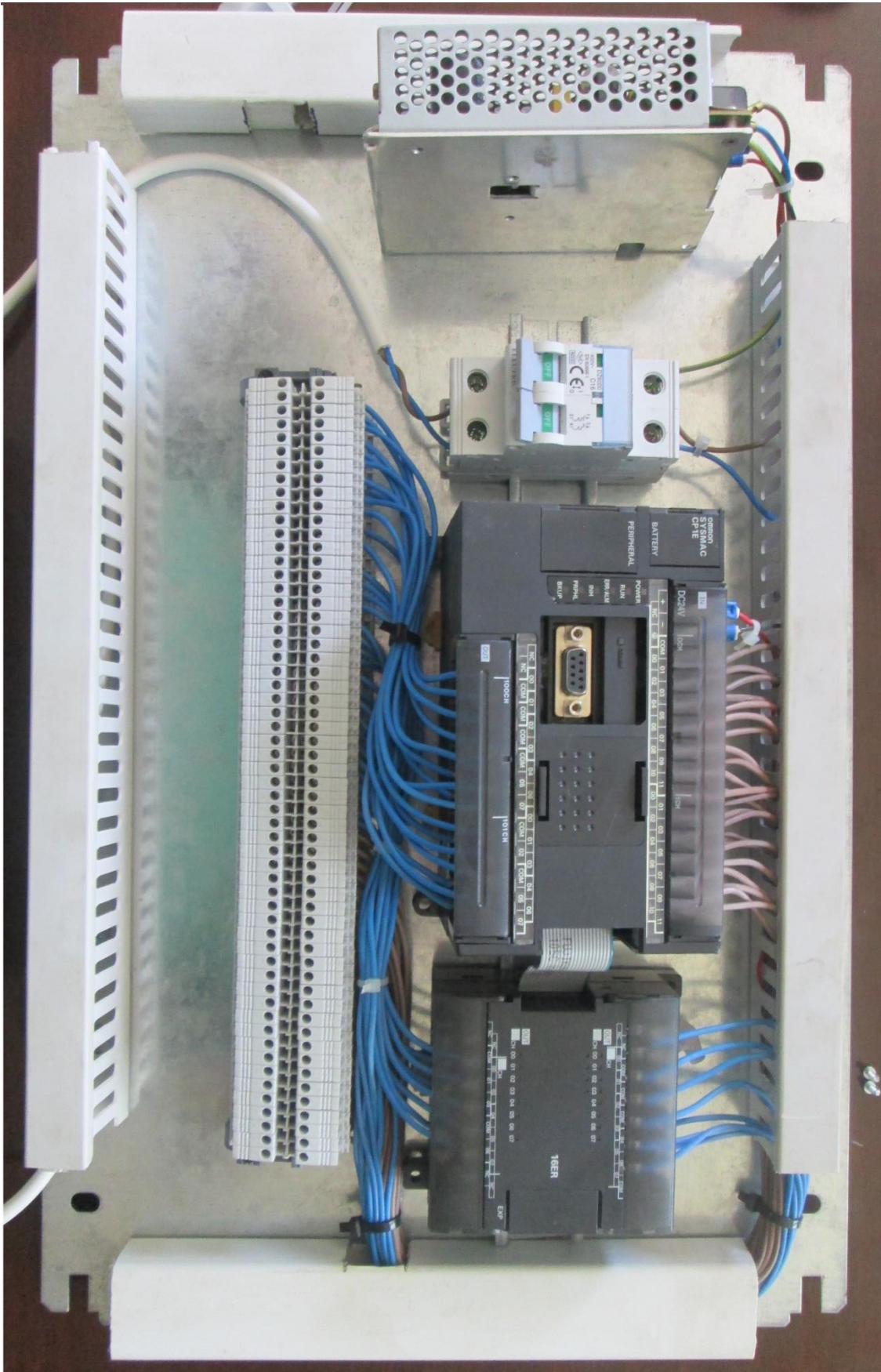
Figure 1.4: the machine's control cabinet.
