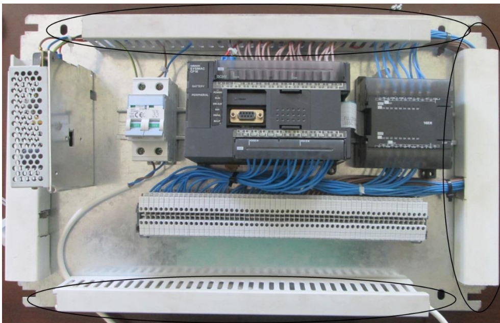
Figure 1.67: open slot panel trunkings with cables.
