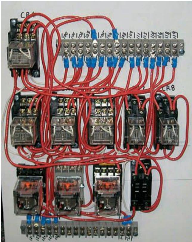
Figure 1.10: Relay based control panel.
