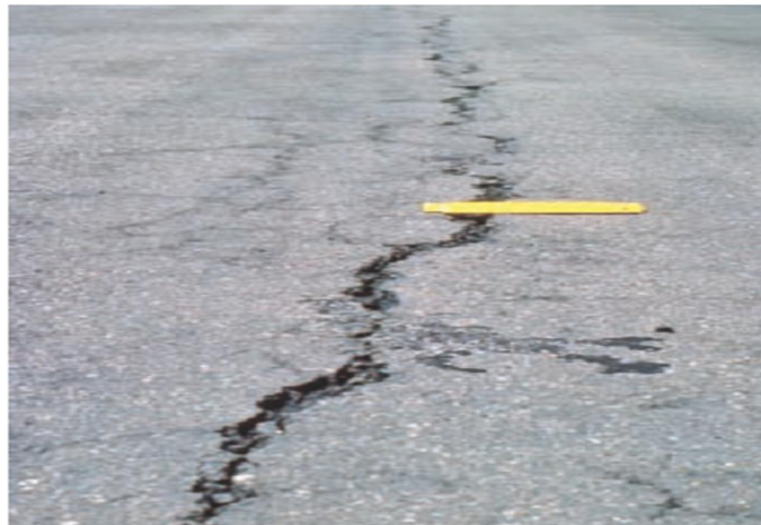
Figure II.6 : Fissure de fatigue
