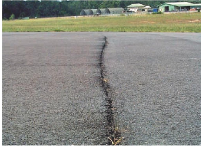
Figure II.8 : Fissure de joint
