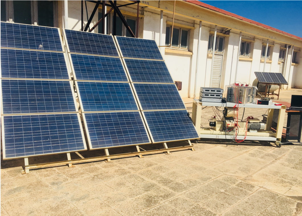
Figure 4.16: Components of PV system under test.
