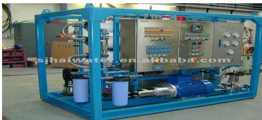
Figure II.4 : La pompe haute pression (PHP)
