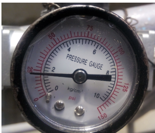
(a) pressure on the compressor barometer
