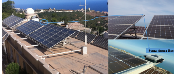
Figure 3.3: overview of the plant in the roof of the lab
