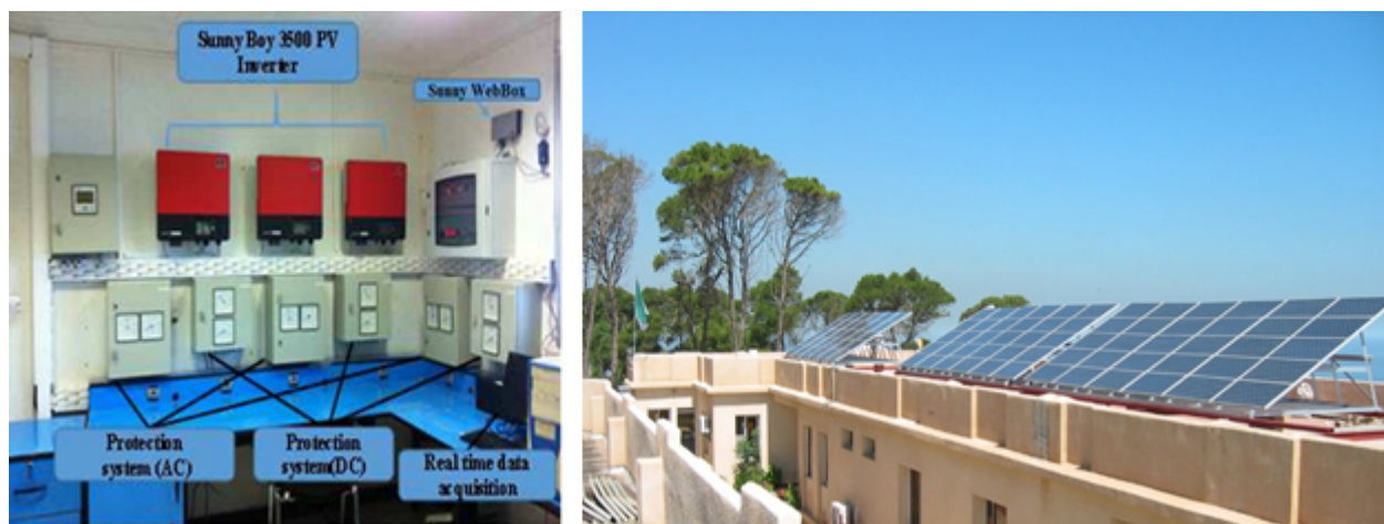
Figure 3.2: An overview of the control room and sub-array.
