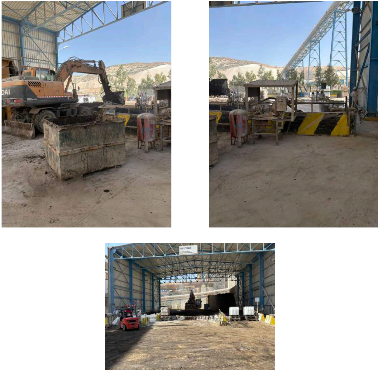
Figure 1.8. The Sludge Treatment Station. (a) An excavator homogenising the incoming sludge; (b,c) the storage basins from which the ASF stream is drawn.
