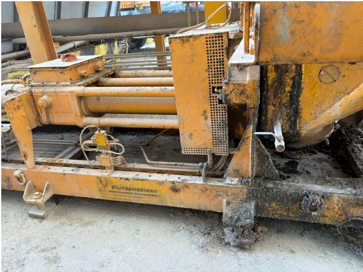
Figure 3.3. The positive-displacement pump that injects the alternative-fuel stream into the calciner.
