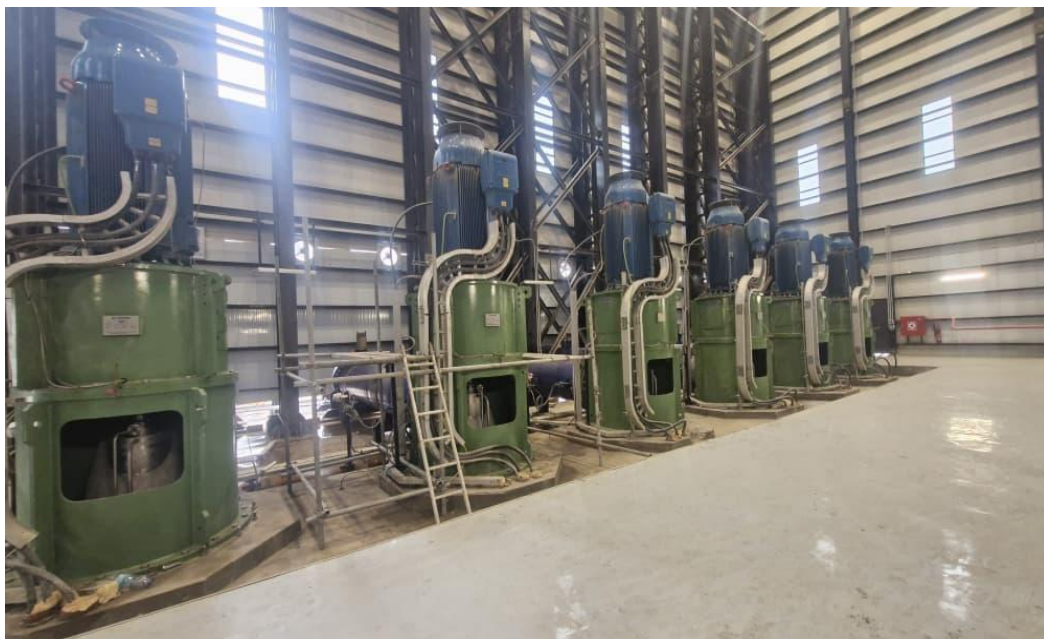
Figure II.5 : Station de relevage (photo originale).
