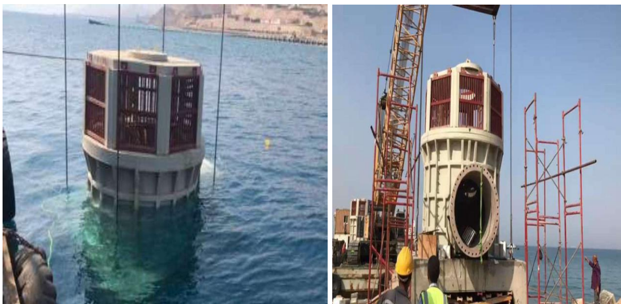
Figure II.2 : La tour de captage (photo originale).
