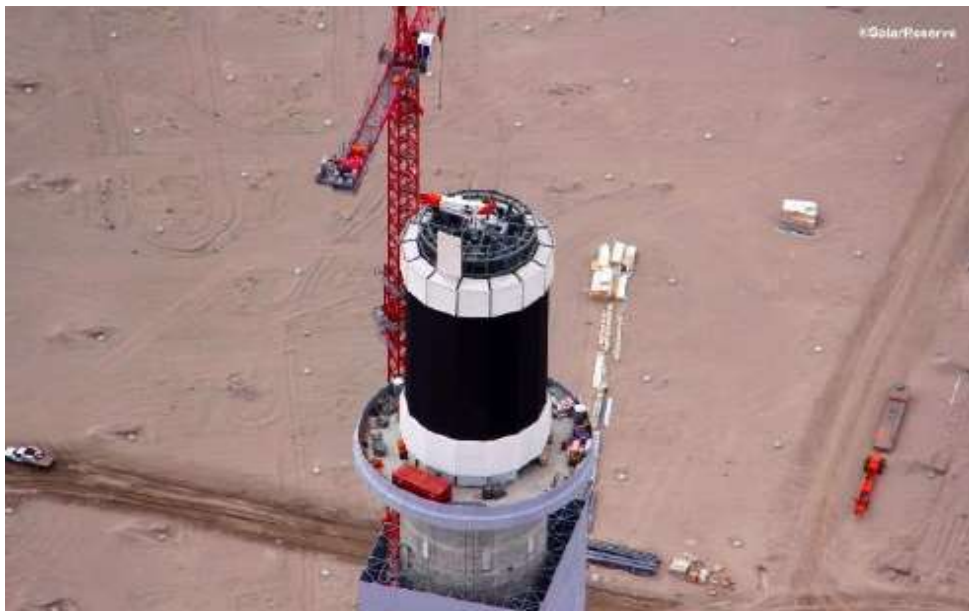
Figure 1.15. External Cylindrical Receiver used in Crescent Dunes Power Tower [57]
