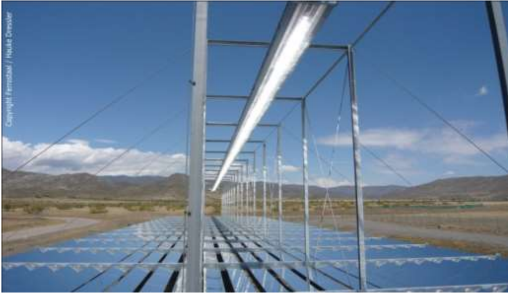
Figure 1.4. 1.4 MW Puerto Errado 1 Thermosolar Power Plant (PE1) at Calasparra, Spain [45]
