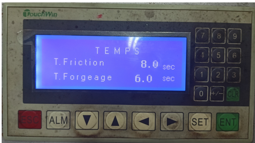
Figure 4.5: The operator control panel
