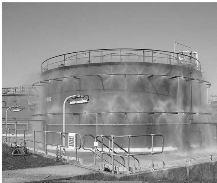
Figure 1.14: Deluge system cooling a storage tank
