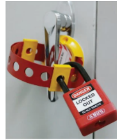
Electrical panel lockout
