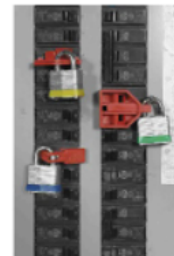
Single pole breaker lockout
