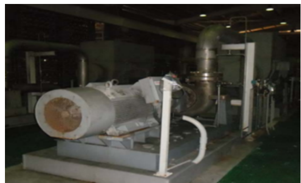
FIG. 3.11: Pompe Booster(Rapport Final de Fouka 1)
