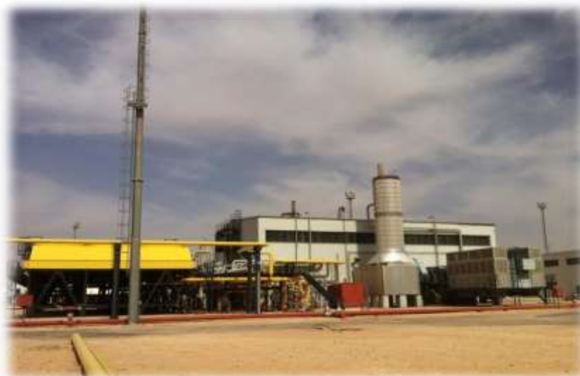
Figure 1.2 : Station de compression de gaz SC1
