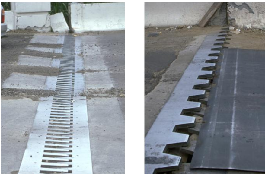
Figure I.11. Joints de chaussée endommagés "Taiwan 1999" [5]
