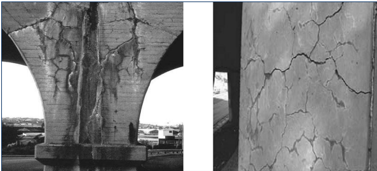
Figure II.1. Fissuration du béton
