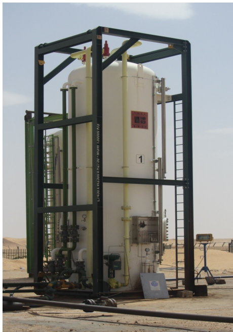
FIGURE 7.5 – Le Surge Tank du champs HGA
