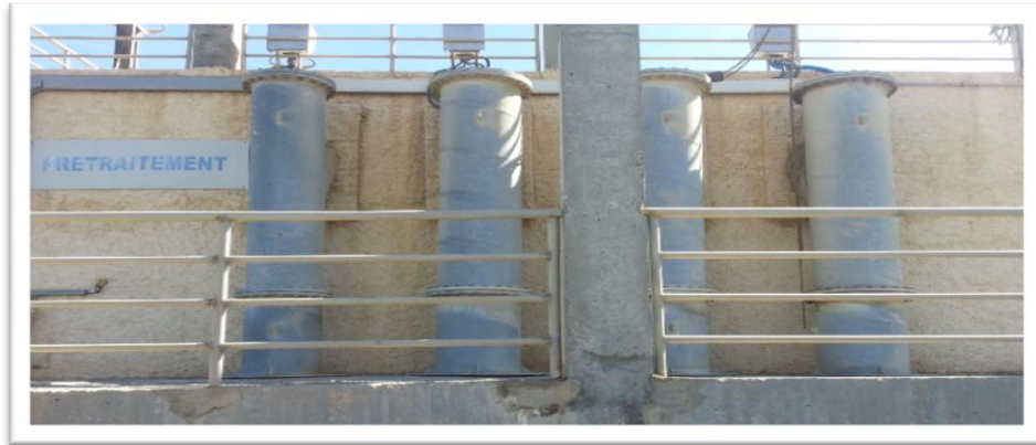
Figure IV.6 : Station de relevage.
