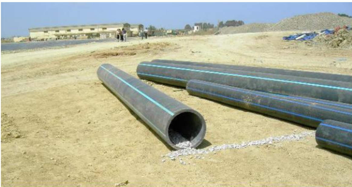
Figure VI-12 : Tube de drainage
