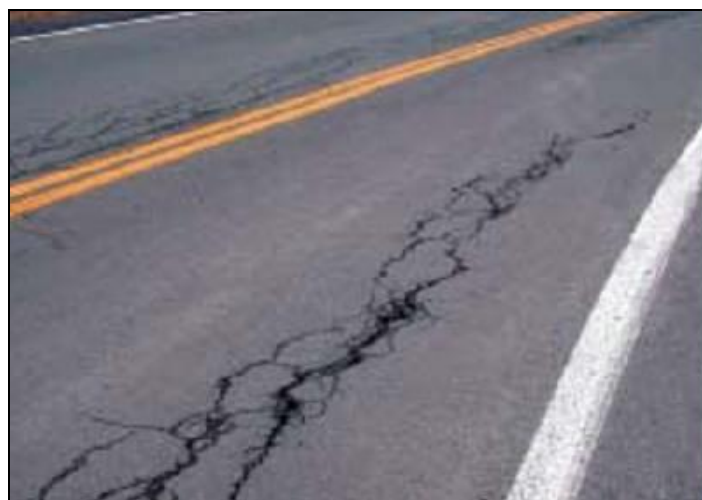
Figure I.5. Fissures de centre
