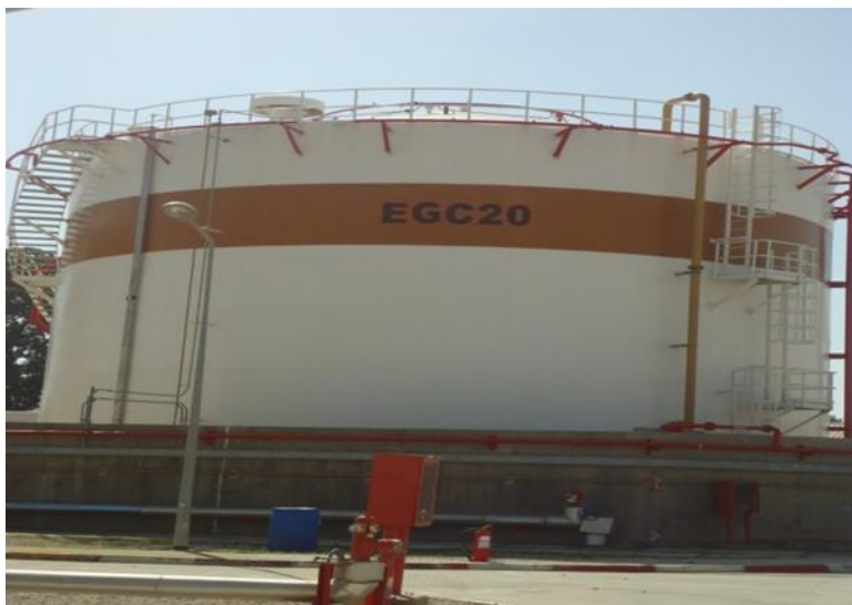
Figure1.6:Bac de stockage fuel EGC20
