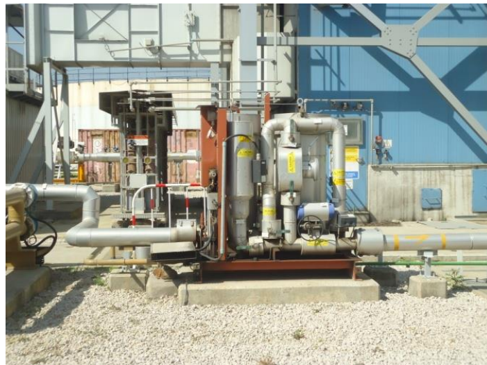
Figure 1.8: SKID de filtration.
