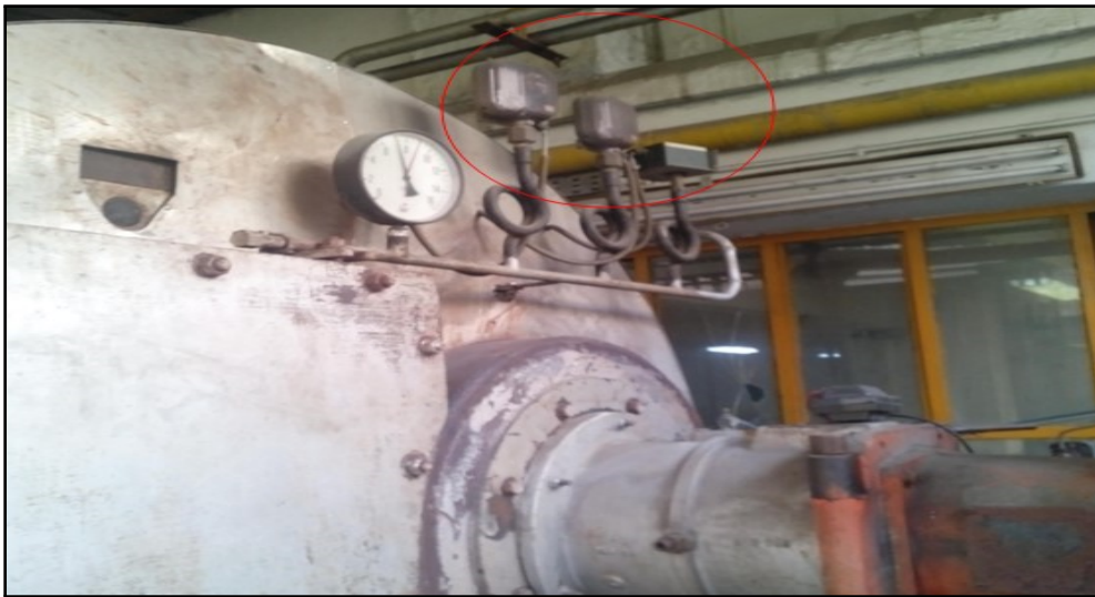
FIGURE 3.23 – Pressostats de la chaudière [Source exclusive]
