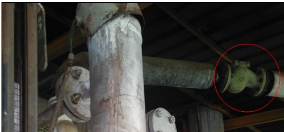
FIGURE 3.22 – Clapet anti-retour de la chaudière [Source exclusive]
