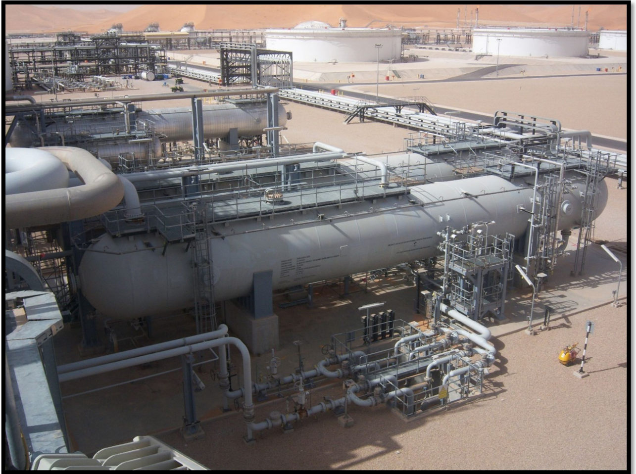
Figure 18: Slug catcher "oil secondary separator V08-1001-3"
