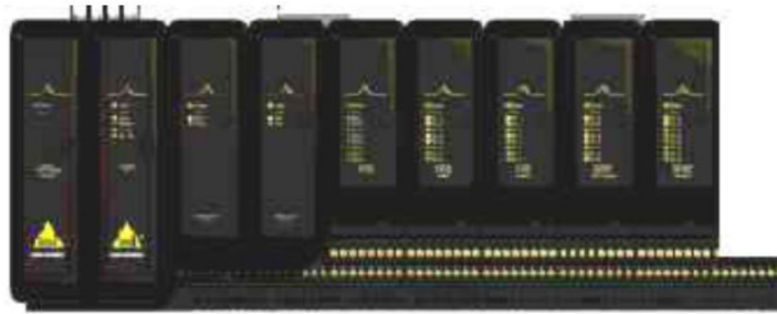
Figure 8: Automates DCS (Digital Control System)
