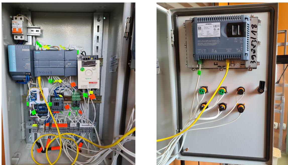
FIGURE 2.2 – Câblage de la station
