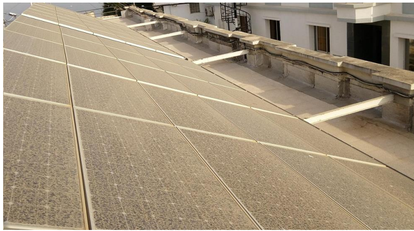
Figure 4.34 PV modules with dusty surface.
