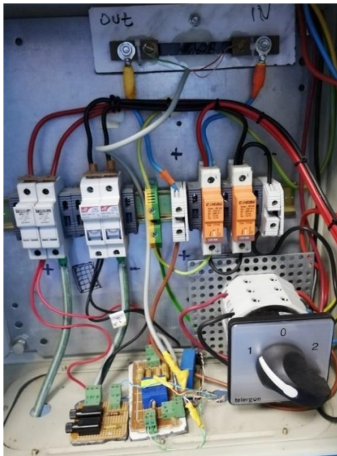
Figure 2.22 mounted sensors on DC cabinet.
