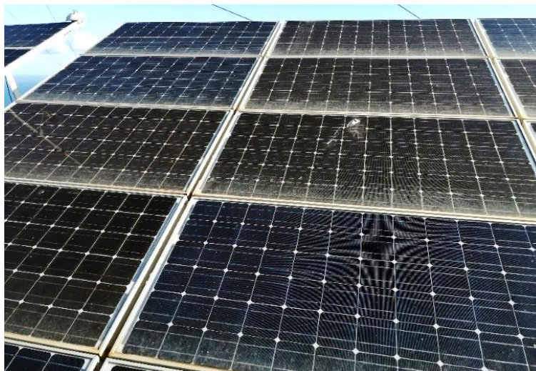
Figure 4.7 Dust accumulation and bird dropping on PV subarray 1.
