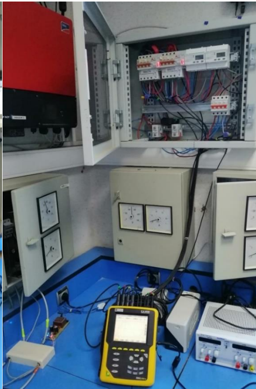
Figure 2.76 C.A 8335 installed on load-lab.
