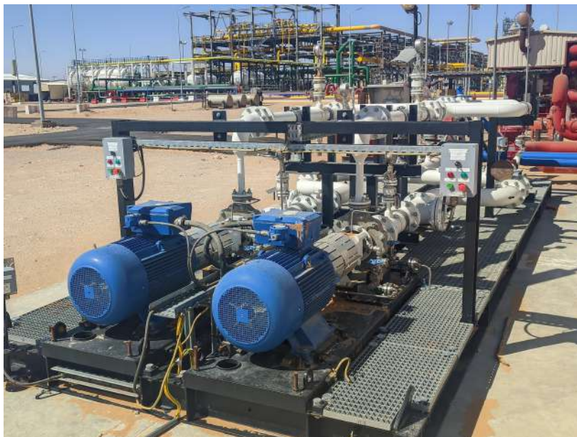
FIGURE 2.3 – Pompes eau de service ( P-4601A/B)
