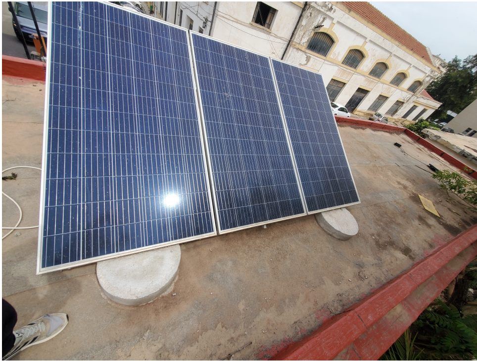
Figure C.1 : The PV array installation
