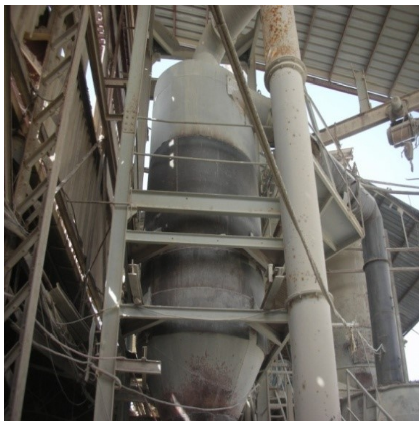
FIGURE 3.14 – Silo de stockage
