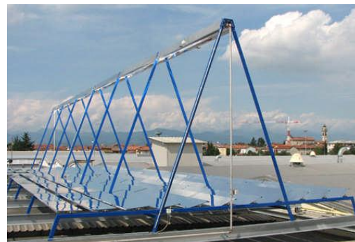
Figure 1.5 Fresnel collector driving an Ammonia-water-chiller in Bergamo, Italy
