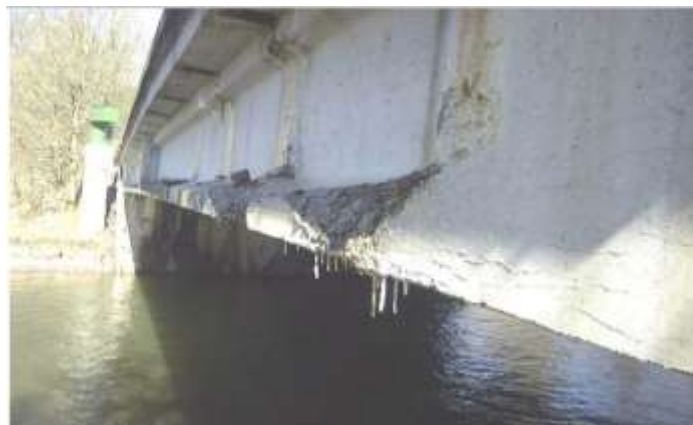
Figure I-6: Fissuration due gel/dégel
