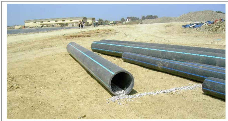
Figure V-8 : Tube de drainage
