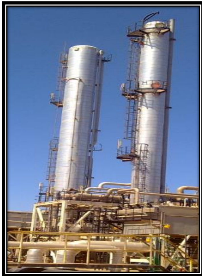
Figure III. 8 : Colonnes de distillation V601 et V602
