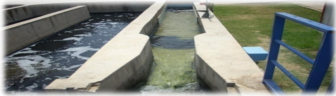
Figure II.9: Bassin de chloration
