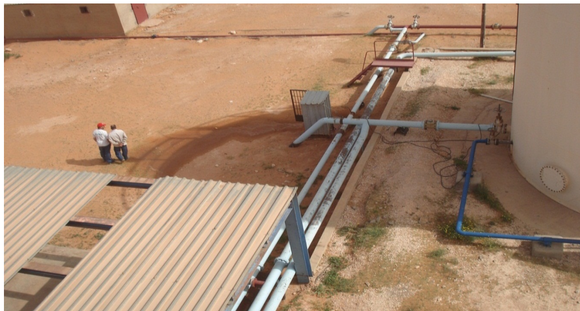
Figure III. 1: la station de pompage nord SP127
