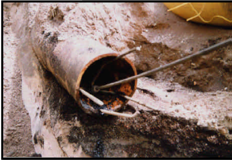
Figure II-3 : Tringlage (Source AXEO)
