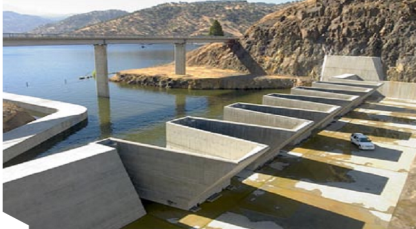
Figure III.11 : hausse fusible labyrinthe
