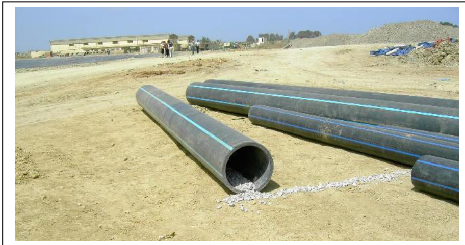
Figure V.12 Tube de drainage
