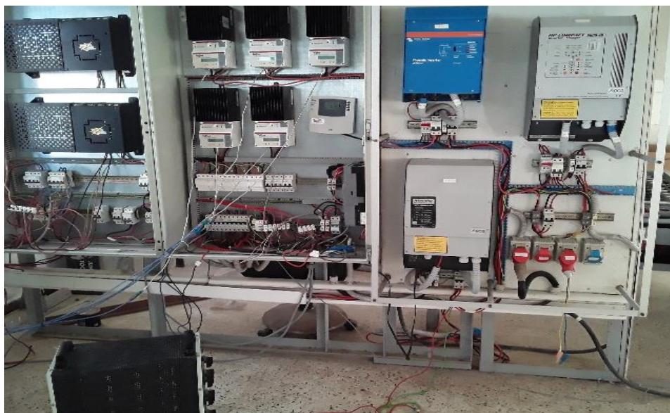
Figure 4.38 Multi-Sources installation (PV / Wind turbines) of the SMS laboratory.
