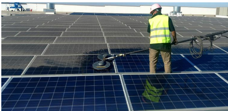
Figure 2.20 Example of PV cleaning.
