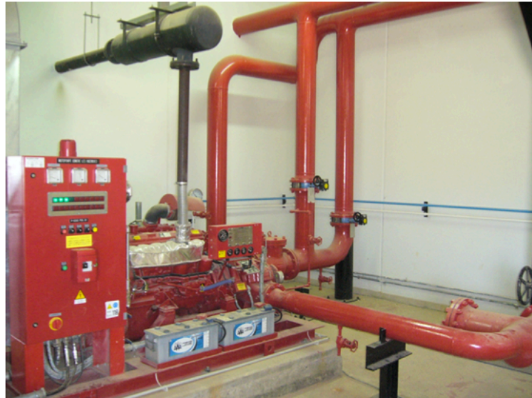
Figure 2-5 : Pompe diesel incendie.[3]
